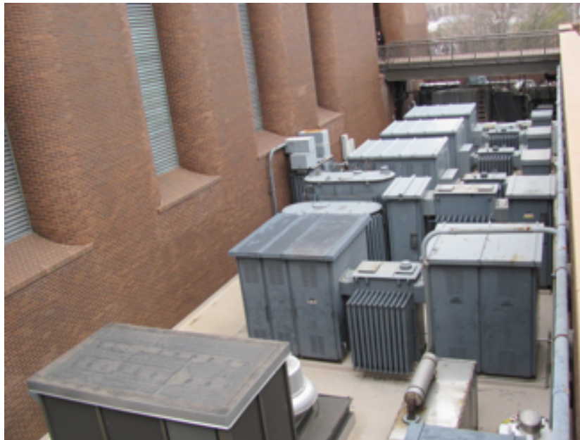
Figure 4.4.4: The Wilson Lab fourth-floor transformer pad
