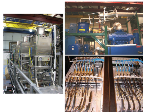
Figure 2: Left: 120 kW CW klystrons. Right, top: Cryogenic pumps. Right, bottom: LLRF control hardware.
